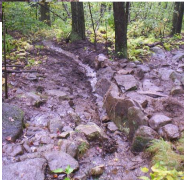
Mike and Tom installing a rock waterbar (above); and a new waterbar doing it's job –Miller State Park, September 2011 work day
