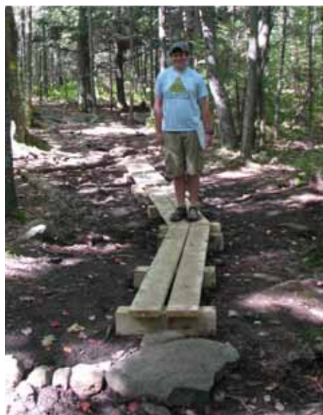
Freddy Wheeler stands on some of the bog bridges he built and installed on the Wapack Trail for his Eagle Scout project.
