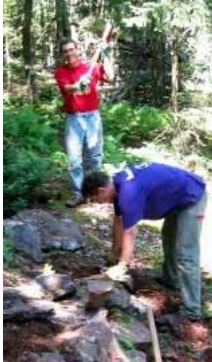
Tom and Mike having fun while building the Spruce Knoll Trail on Pack Monadnock, New Hampshire Trails Day, 2003.
